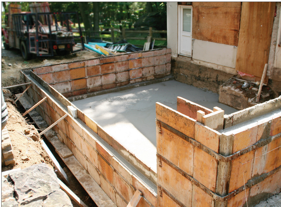
IF NOT properly addressed, ground water can affect an existing foundation and the ability to build successfully.
