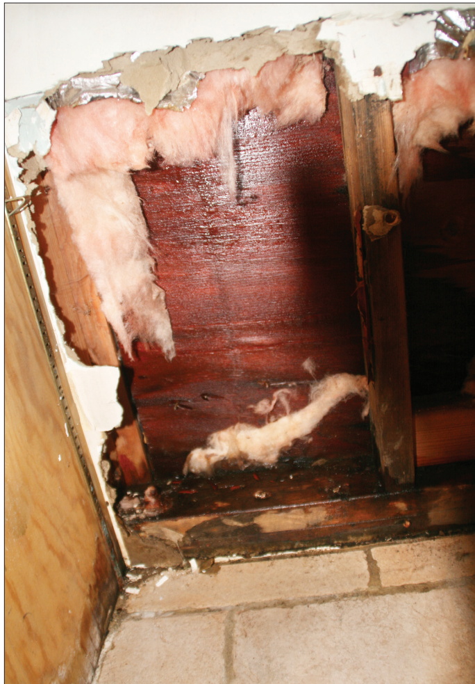
HOMEOWNERS OFTEN discover hidden problems when delving into renovations. Budgeting for remediation can help remove some of the stress of unexpected delays and concerns.
